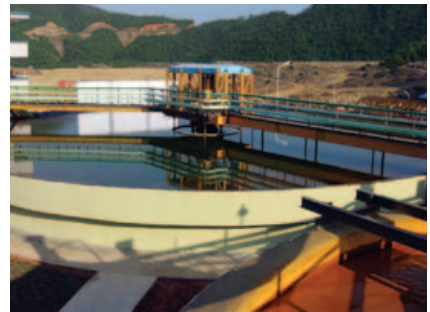
BioteQ's Dexing operation removes dissolved ferric iron and copper from wastewater.
